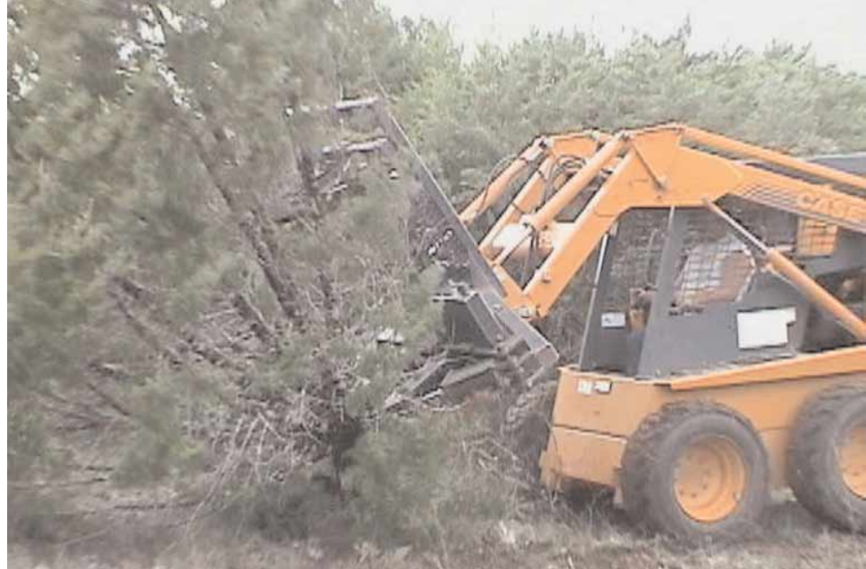
Skid-loader being used to clear juniper at the Leon River Restoration Project.
